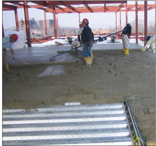
No rebar or mesh to pull up
