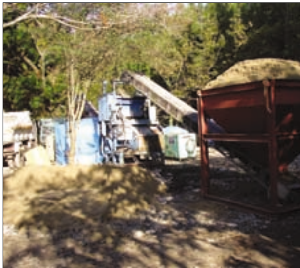
Mobile batch plant
